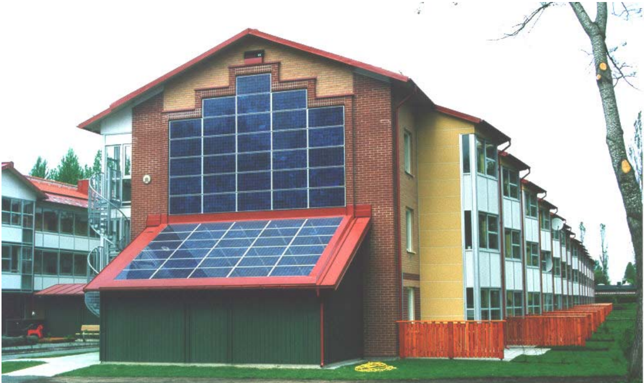
Solar modules were mounted on a residential apartment's building gable in a renovation project.
