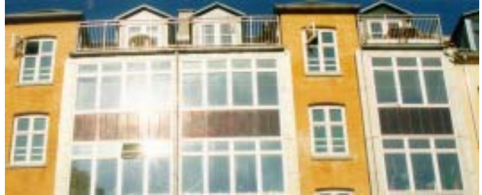
Solar modules can replace conventional building materials and be true parts of the building structure. In this renovation project, part of the balcony wall is covered with solar modules.
